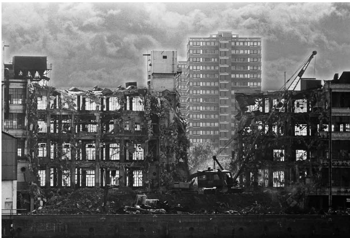
Demolition of the Morgan Crucible Factory in Battersea, 1979, by Sarah Wyld who will be showing photographs (1970s to the present day) during Wandsworth Artists Open House 2012
